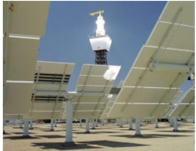
Warren Gretz, NREL/PIX02157
