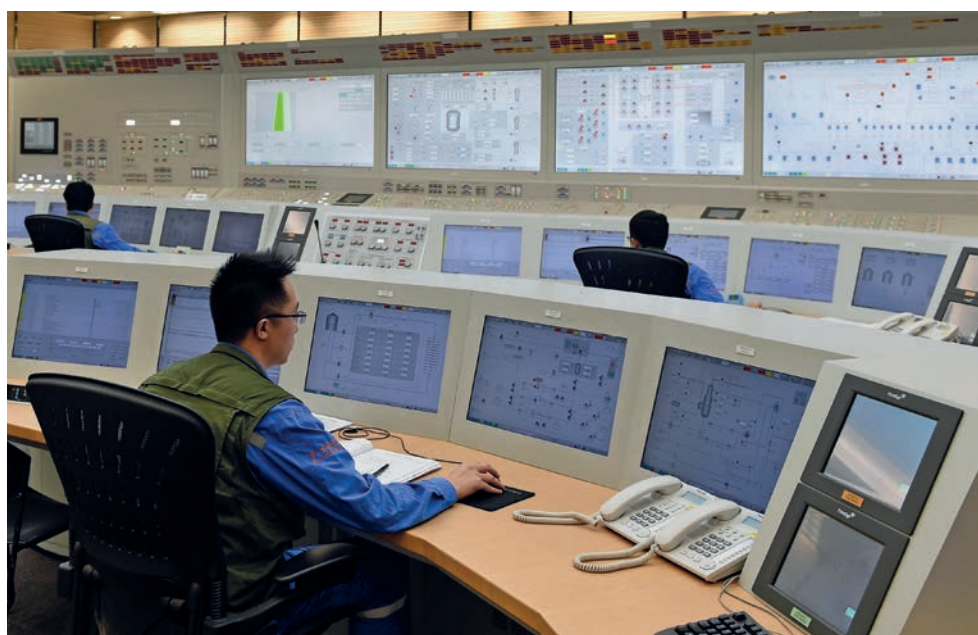
Yangjiang 5 control room (Image: Yangjiang Nuclear Power Co)
