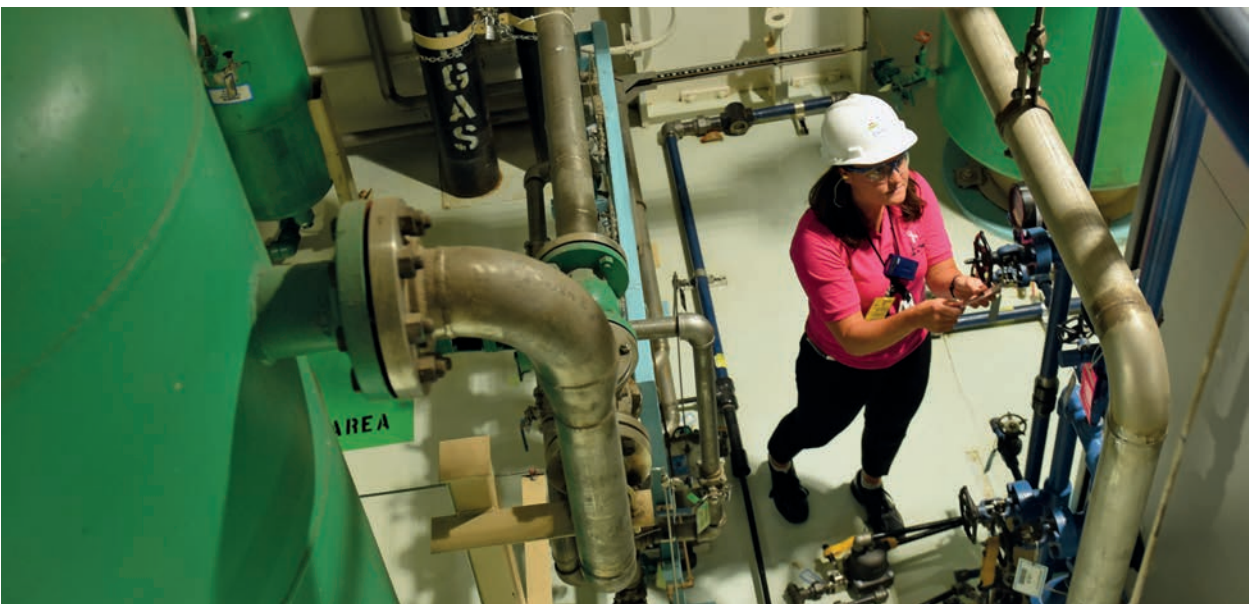
Sarah Coady, Design Engineer, examines the Instrument Air System at Dresden 3 (Image: Exelon)
