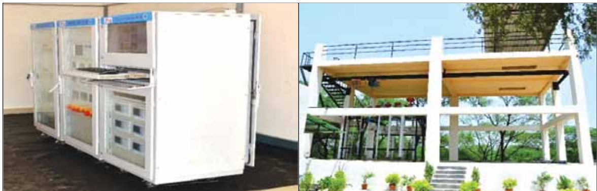
Fig.7.12: Solar Water Pump Facility for up to 50 hp capacity
