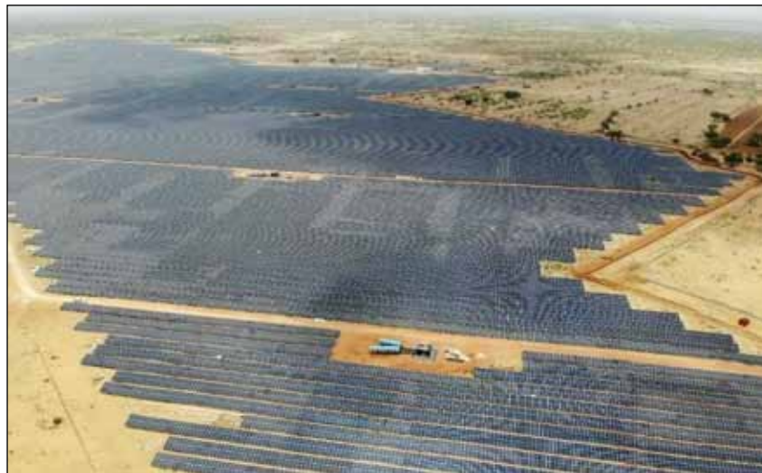
Fig. 10.31: 300 MW Solar Project in Jaisalmer, Rajasthan under SECI-IV tender
