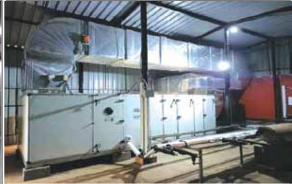
Fig. 7.11(b): Required infrastructure to be installed in the LDSR facility to achieve Class 10000 specifications of the clean-room
