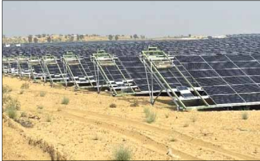
Fig.10.30: 2x300 MW Solar projects in Rajasthan under SECI (ISTS-I) tender
