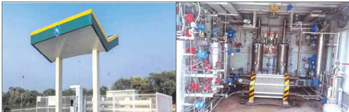
Fig. 10.5: (Left) Solar PV based Green Hydrogen production-cum-dispensing facility at NISE (Right) Installation of new electrolyser at NISE Hydrogen generation facility
