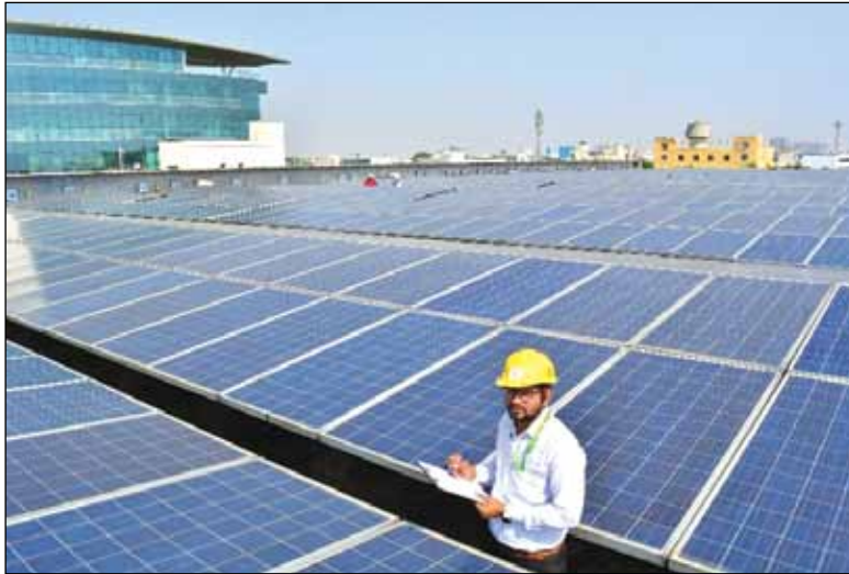
Fig. 10.13: Testing Services by NISE Technical Team at Roof Top Solar PV power plant, Manesar
