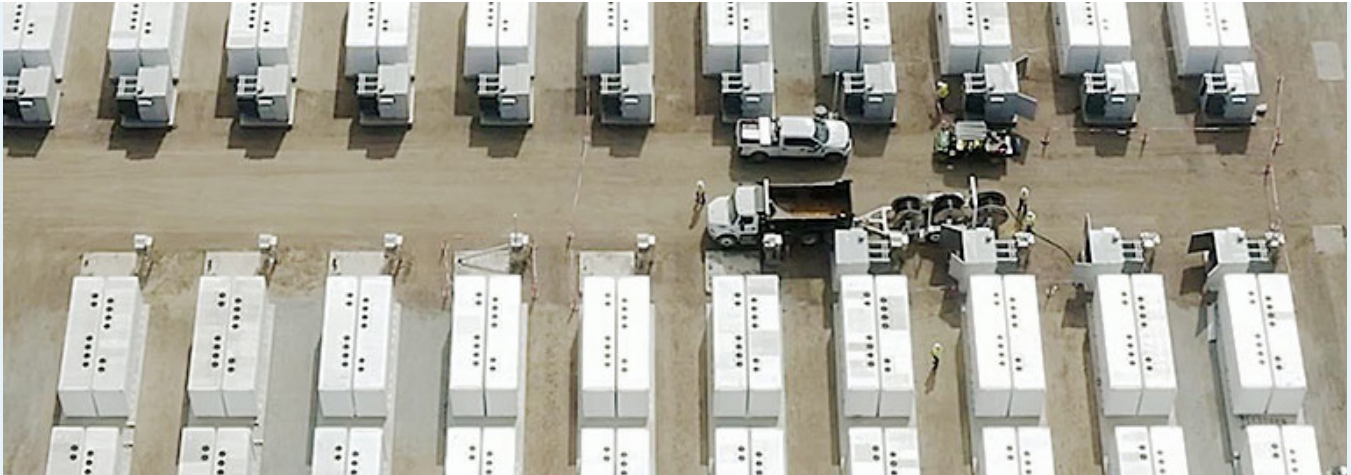
Photo of PG&E's Elkhorn Battery in Monterey County, a 182.5 MW battery energy storage system that is one of the largest utility-owned, lithium-ion battery energy storage systems in the world.
