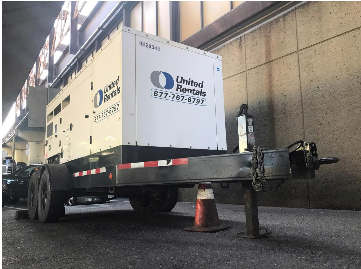
Figure 15. Portable Generator Adjacent to Rockridge Station
