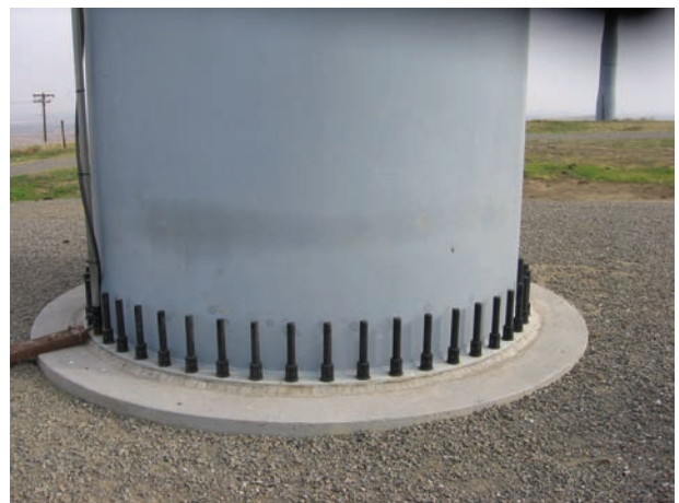
Base of Diablo Winds Vestas V47 Turbine (Pier Foundation)
