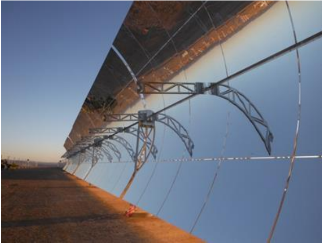
NOORo I construction site – Erection of the parabolic reflector. Source: KfW / Jesús Vazquez Serrano, ARIES INGENIERA Y SISTEMAS, S. A.
