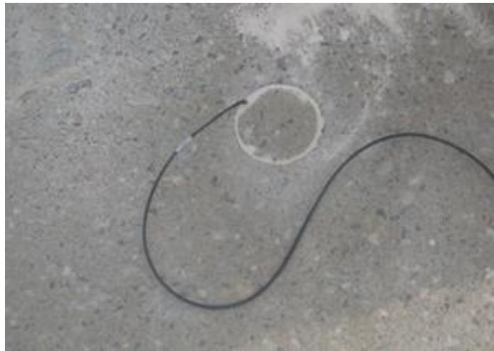
Figure 40. Installed heat flux sensor with cap cover
