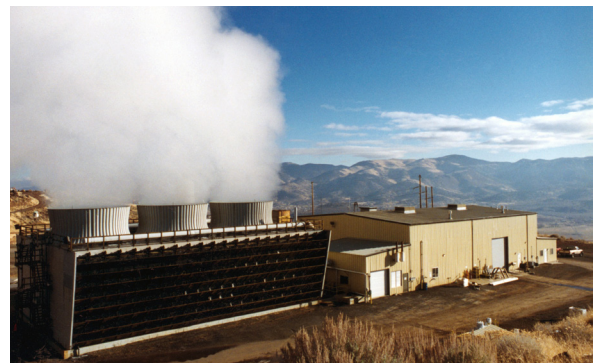
Steamboat Hills Geothermal Power Plant 31 Steamboat Springs, Nevada
