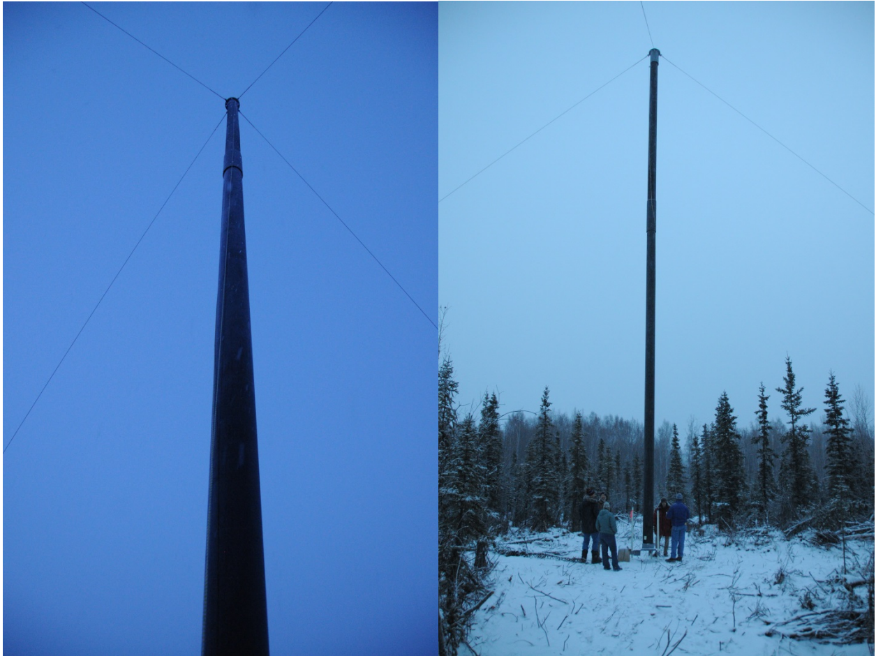
Figure 8: GFRP Pole as Installed
