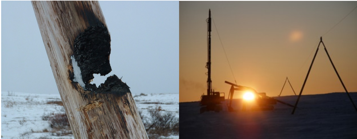
Figure 10: Failed Pole Support Due to Lack of Grounding and Lack of Fault Detection (left, source: Alaska Industrial Development and Export Authority). New Bethel–Napakiak 3-Phase AC Intertie Under Construction (right, source: Denali Commission).
