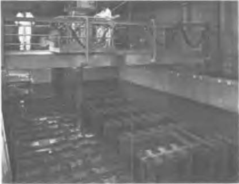
FIG.11a. WAK pool, Karlsruhe, Federal Republic of Germany, showing stationary stainless steel and aluminium fuel storage racks.
