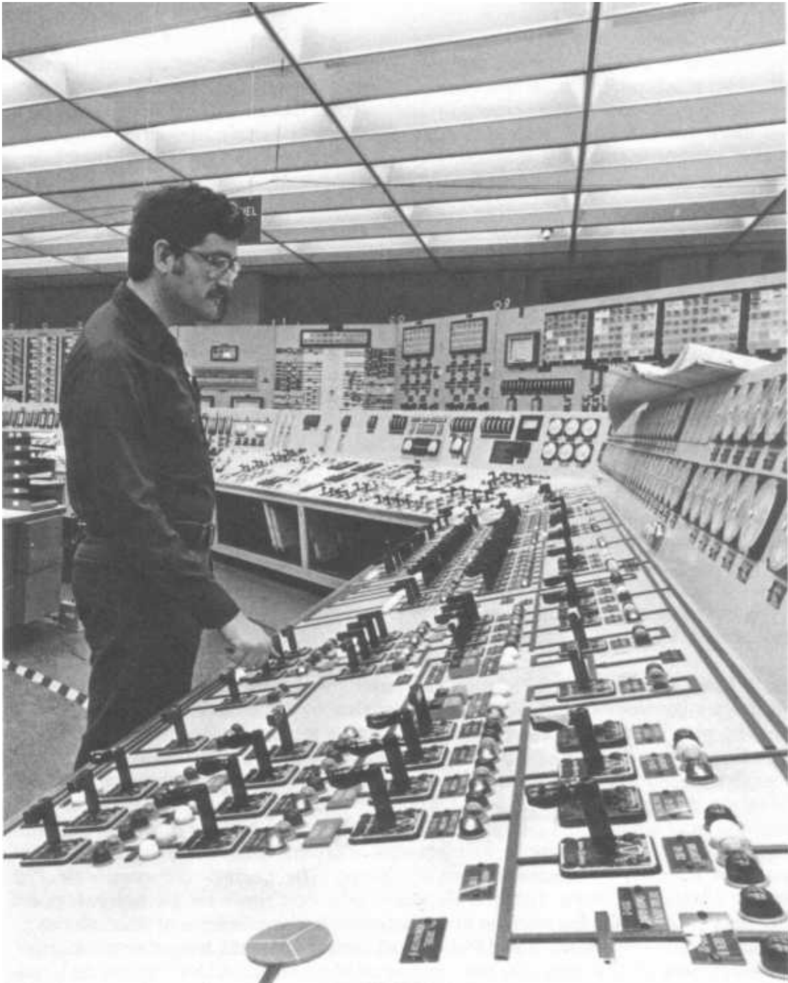
The size and layout of the Unit 2 control room may have contributed to the operators' difficulties in responding to the accident.
