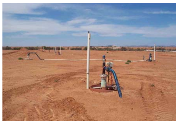
Figure 5 Active extraction wellfield at Beverley
