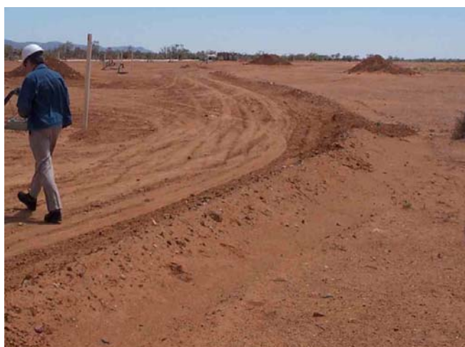
Figure 14 Example of earthen bund, around Beverley wellfield
