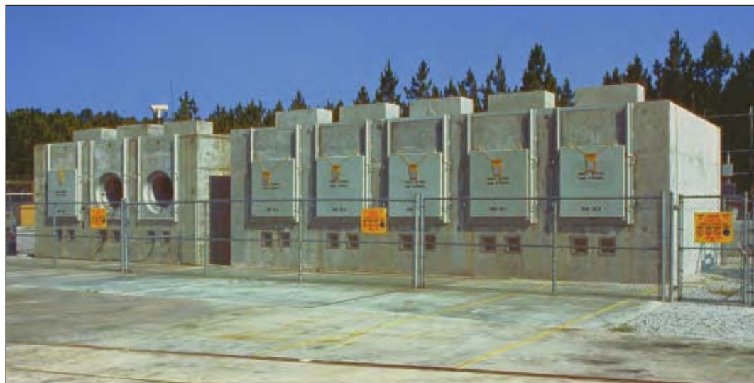
Figure 4.3 Independent Spent Fuel Installation - Dry Cask Storage
