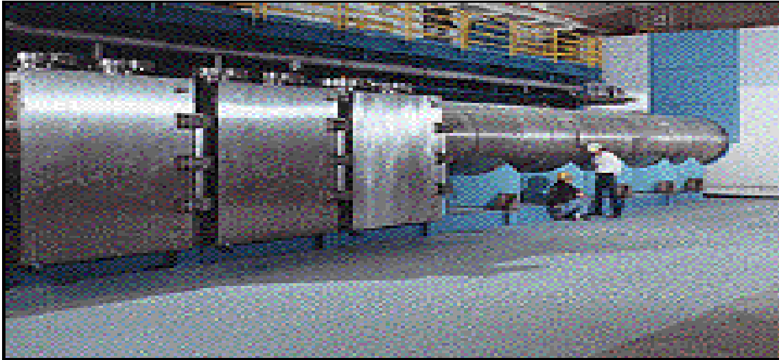
Figure 3-9. Plant-scale Uranium Separator System
