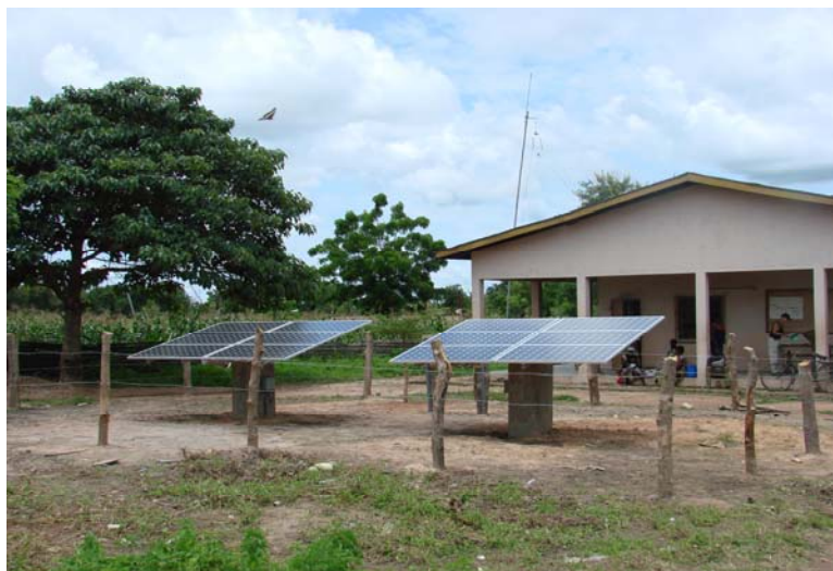
Solar pumping array for Benin Agricultural Project - Benin
