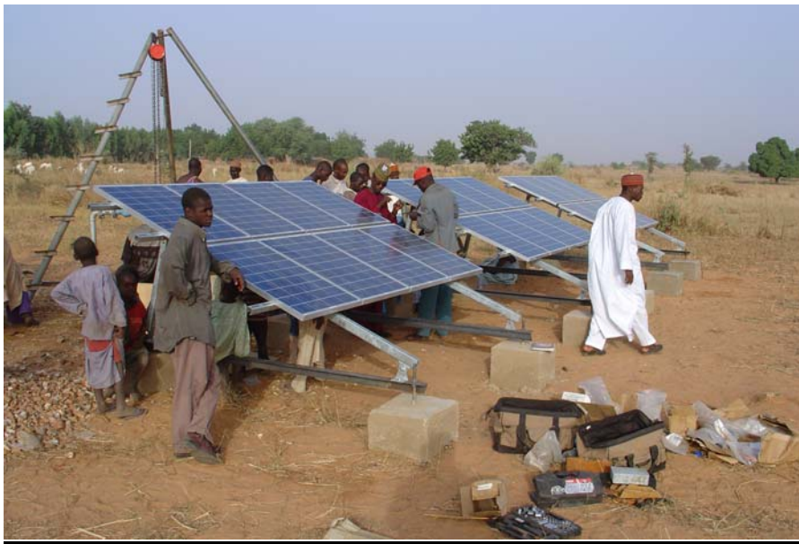
Solar powered village water supply - SELF- Nigeria
