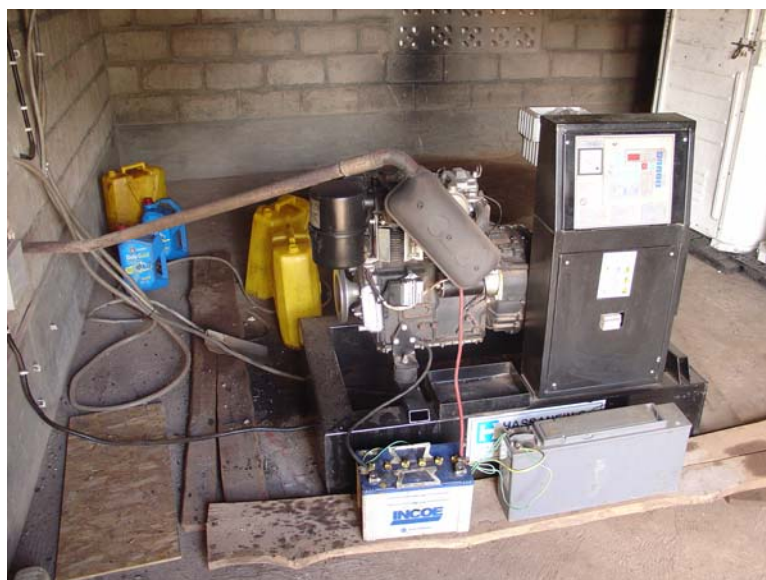
Besides economic and reliability concerns, diesel generators create noise and air pollution and contribute to climate change.
