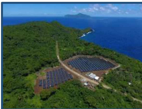
Solar Plant on Ta'u Commissioned in October 2016.
