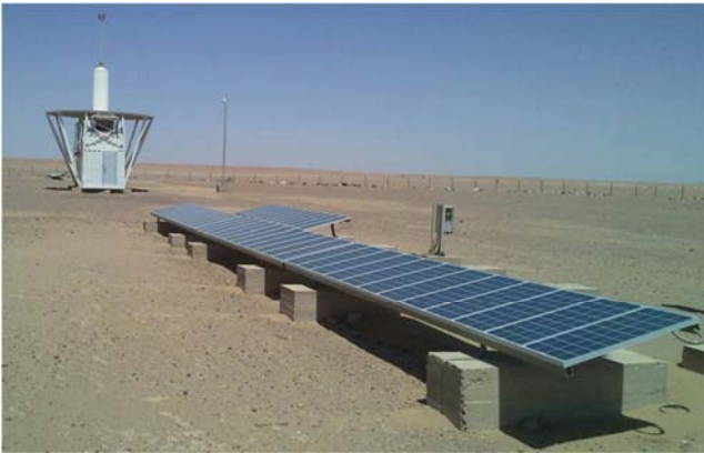
Figure 9. Solar energy system to operate radio navigation station for aircraft in Dongola International Airport.
