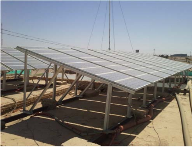
Figure 8. Solar system in Dongola International Airport Aerodrome Control Tower.
