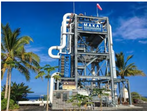
OTEC Pilot Project, Keahole Point, Kona
