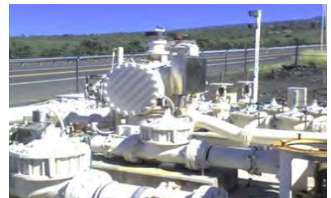
Hawaii County Dept. of Water Supply's 45 kW in-line hydro plant in Kona,
