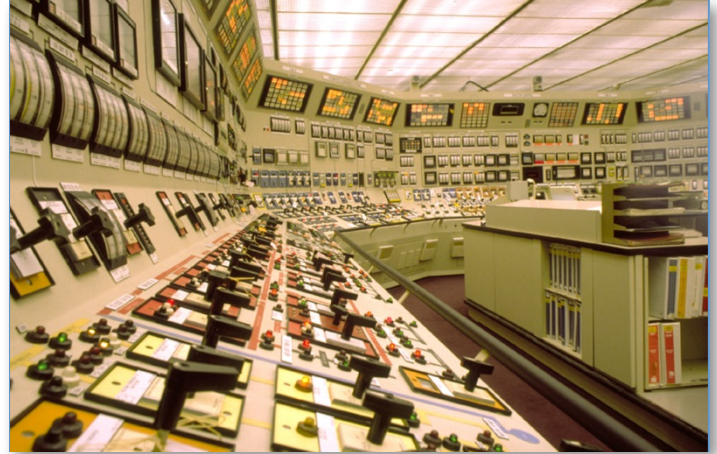
Figure 1. Typical Power Plant Control Room 2
