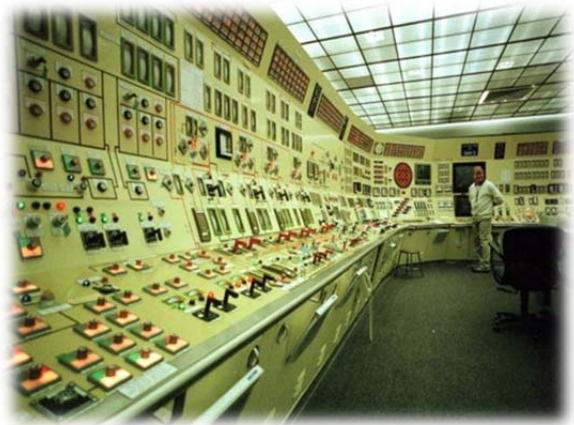
Figure 10. Typical nuclear power plant control room with analog technology.
