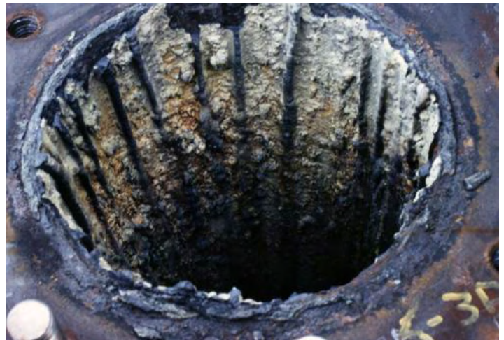
Figure 13 – Scaling and corrosion caused by impurities in hydrothermal fluids are major contributors to high O&M costs for geothermal power plants. (Credit: NREL)
