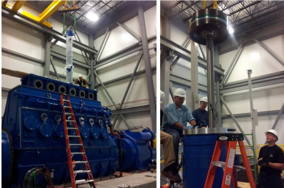
Figure 2: Left: Test-fit of a SustainX HP cylinder on top of the lower-half of a MAN engine (crankshaft). A PMG can be seen to the right of the crankshaft. Right: Installation of a LP piston into a LP cylinder.
