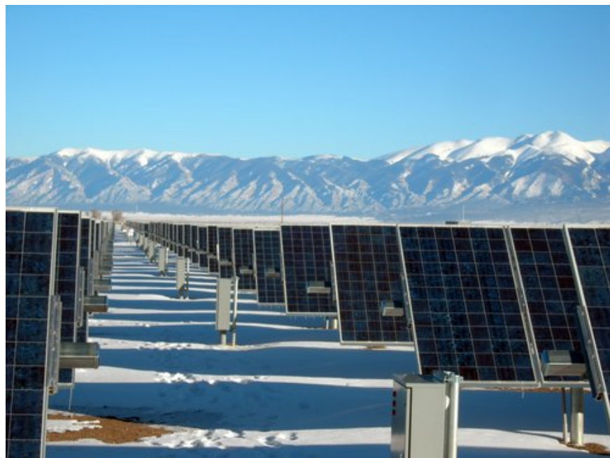
Figure 14. SunEdison's 8.2 MW Alamosa plant
