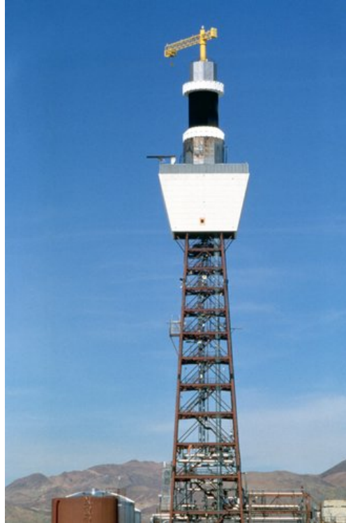
Figure 12. The Solar Two system in California included a thermal energy storage system
