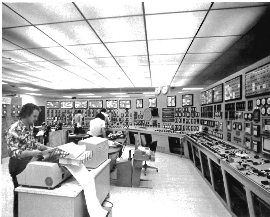
Fig. 6. Control room of a commercial nuclear power plant. A myriad of lights, dials, and switches monitors and controls all the complex systems within the plant. (Photo courtesy of Florida Power & Light Company.)
