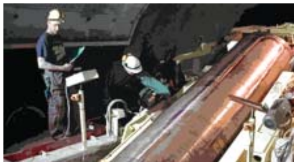
A major 'prototype repository' project in Sweden has tested the engineering methods needed to place full-scale model spent fuel containers into disposal locations in a deep underground laboratory in granite – a dummy (non-radioactive) copper container can be seen being rotated for emplacement in a disposal hole in the floor of a tunnel (courtesy SKB).
