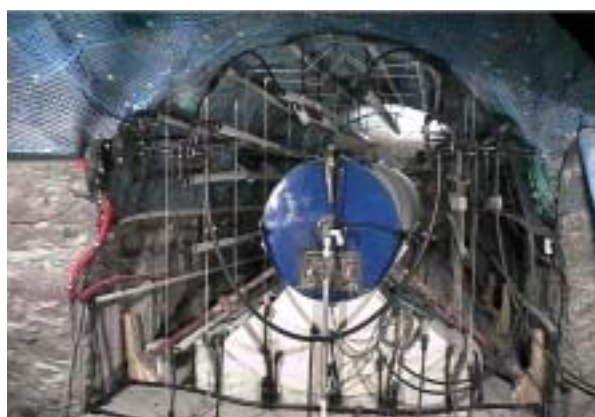
A heated, dummy waste container being emplaced into a tunnel in clay, where it will be surrounded by pelletised bentonite clay buffer material. The container is initially supported on blocks of compacted bentonite (courtesy ENRESA).
