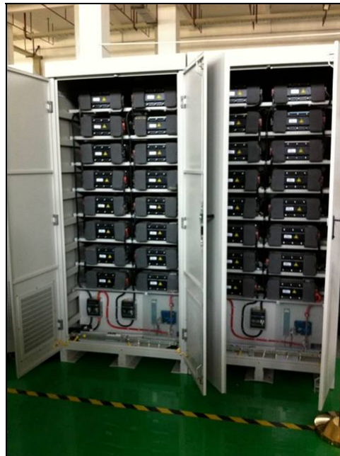
Figure 4-21 A 50-kWh BYD Li-ion Battery System Planned to be Tested at EPRI's Knoxville, Tennessee Smart Grid Laboratory in 2011.
