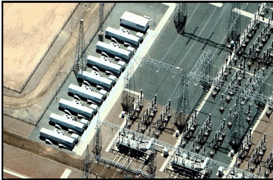
Figure 4-19 Commercial operation of a 12-MW frequency regulation and spinning reserve project at AES Gener's Los Andes substation in the Atacama Desert, Chile. The system uses A123 Systems' Li-ion Hybrid Ancillary Power Units (Hybrid-APUs™).
