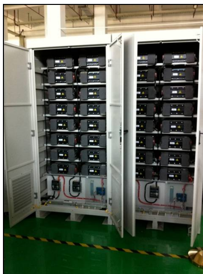
Figure 8 A 50-kWh BYD Li-ion Battery System Planned to be Tested at EPRI's Knoxville, Tenn. Smart Grid Laboratory in 2011.
