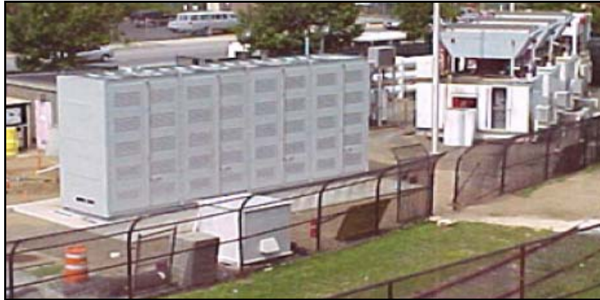
Figure 4-10 NYPA 1.2-MW/7.2-MWh Sodium-Sulfur Battery Facility
