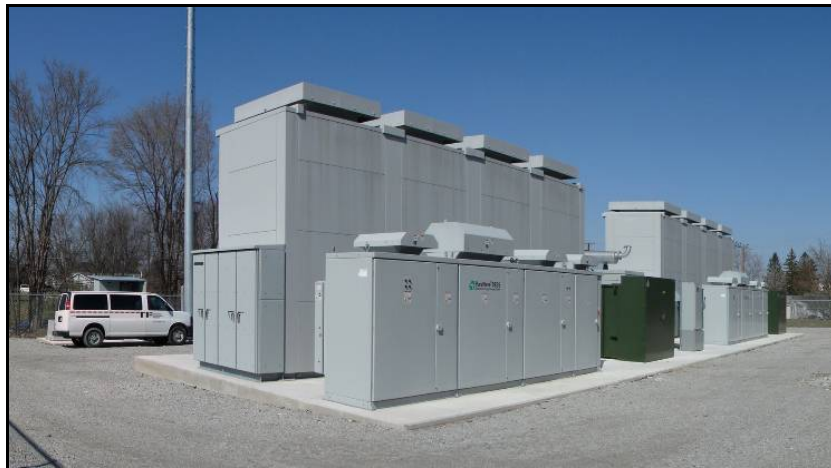
Figure 4-11 AEP Distribution Substation with Sodium-Sulfur Unit
