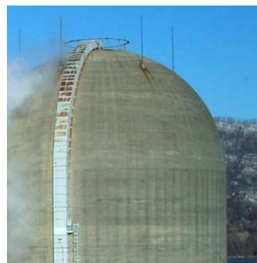
Visible rust on the containment building vents, while having no safety implications, presents the appearance of disrepair.
