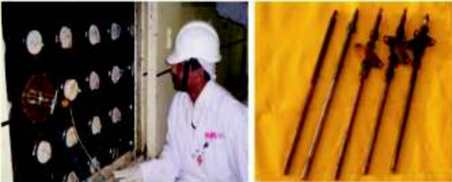
In-situ laser cutting of bellow lip in reactor and 18 mm thick shock absorber studs cut from reactor
