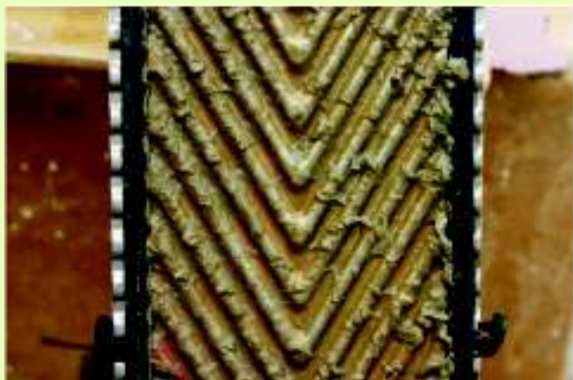
Ti plate heat exchangers with heavy microbial fouling
