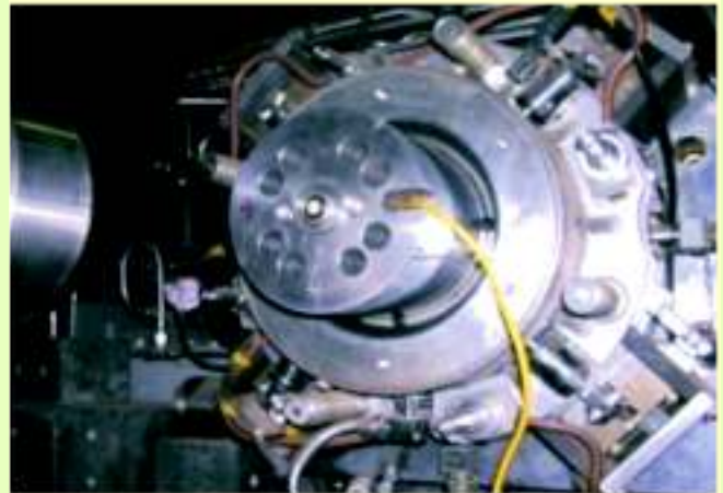
Sensor mounted in Fuelling Machine snout
