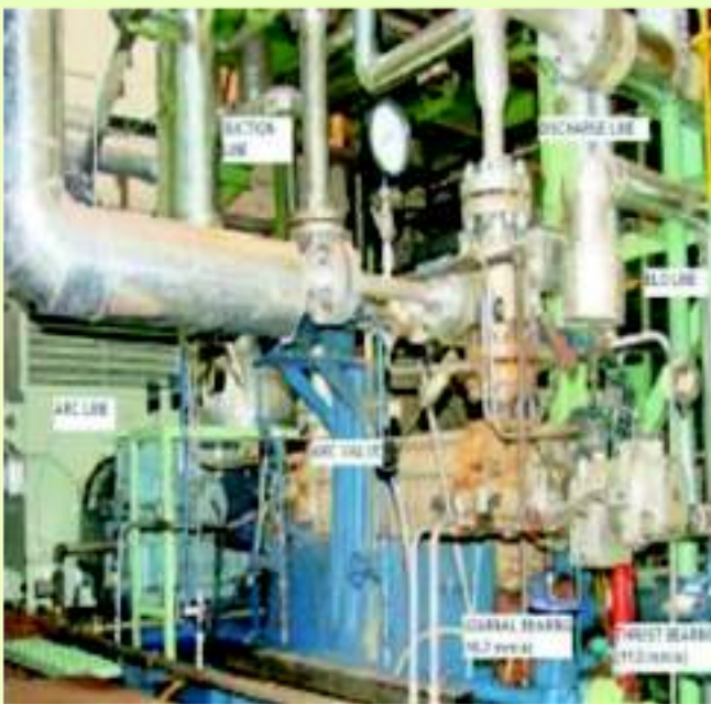
Steam Generator Facility, Kalpakkam
