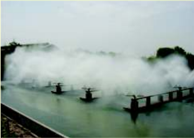
Mist Cooling System Commissioned at Heavy Water Plant, Kota. This system has eliminated requirement of water for dilution of effluent and has resulted in less effluent generation
