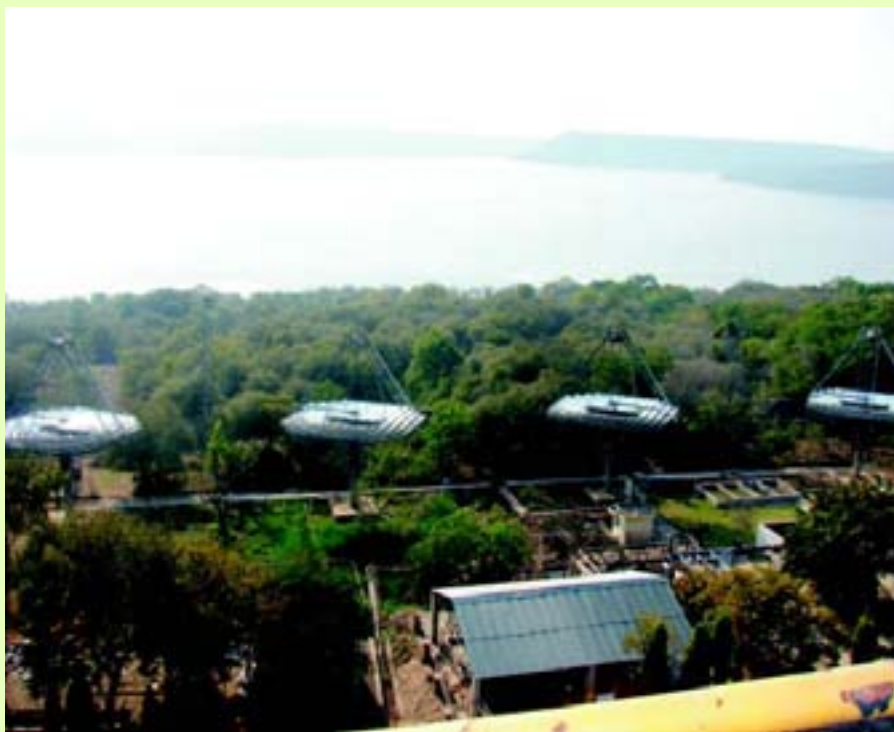
Solar Steam Generator System at Heavy Water Plant, Kota
