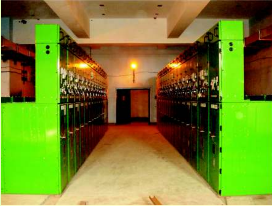
6.6kV Switchgear panels (Bhavini)
