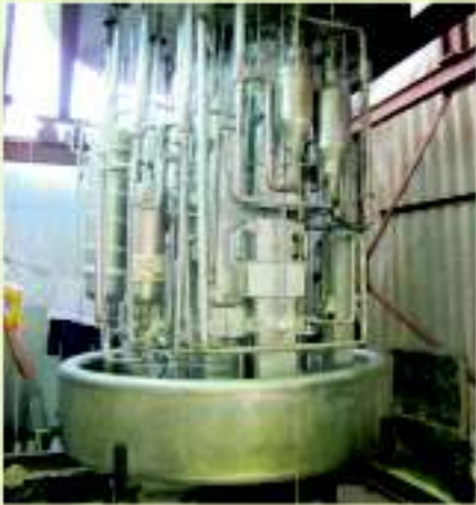
Cold box internal view
