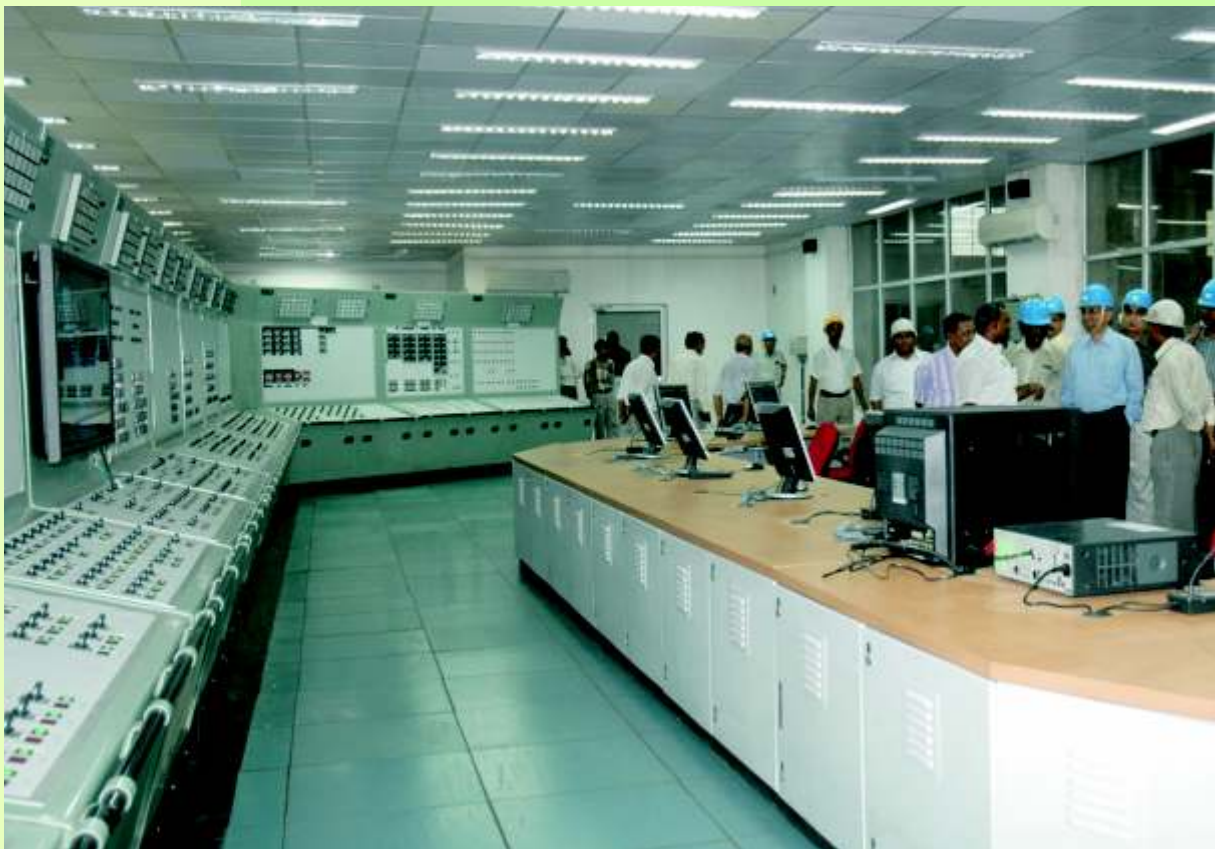
SCADA System developed by ECIL for the Uranium Corporation of India Ltd.
