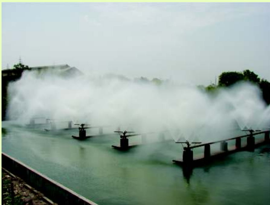
Mist Cooling System Commissioned at Heavy Water Plant, Kota
