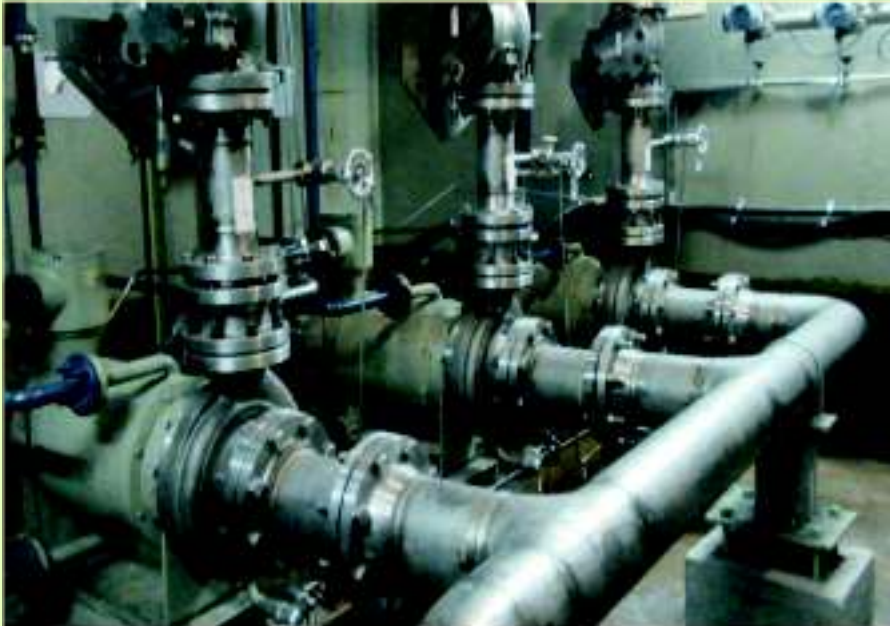
New Emergency Core Cooling System pumps of DHRUVA
