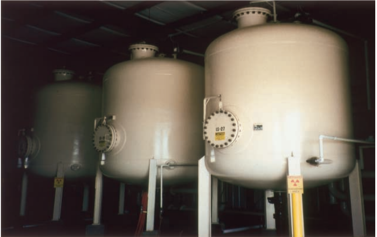
FIG. 33(c). ISL production equipment, Smith Ranch, Wyoming, USA. Columns hold ion exchange resin to recover uranium from leach solution pumped from the wellfield.
