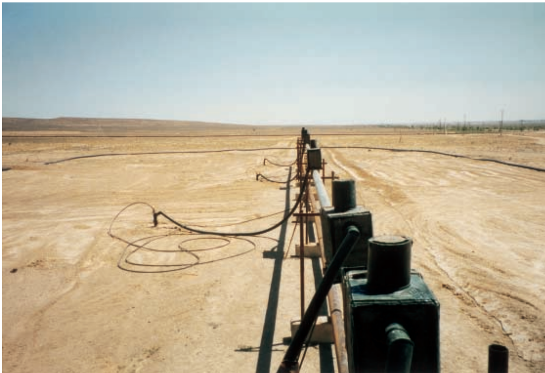
FIG. 32(b). ISL wellfield, Zarafshan, Uzbekistan. Close-up of row of production wells.
