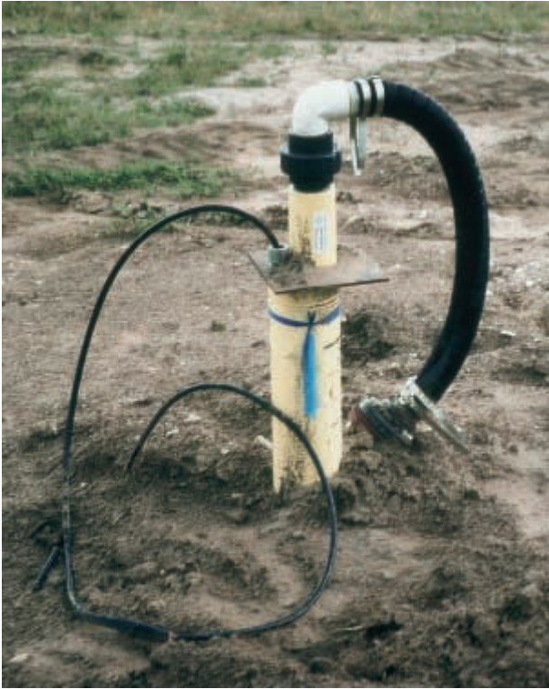
FIG. 33(a). ISL production equipment, Wyoming, USA. Newly constructed production well.
