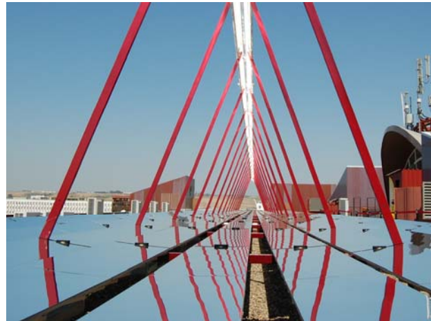
Figure 5.12 Fresnel process heat collector in operation
