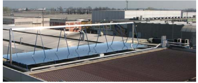
Figure 5.9 PSE Fresnel process heat collector powering two NH 3 /H 2 O absorption chillers (2006, Bergamo, Italy)
