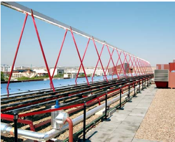
Figure 5.11 Fresnel process heat collector on the roof of Escuela Técnica Superior de Ingenieros, Sevilla
